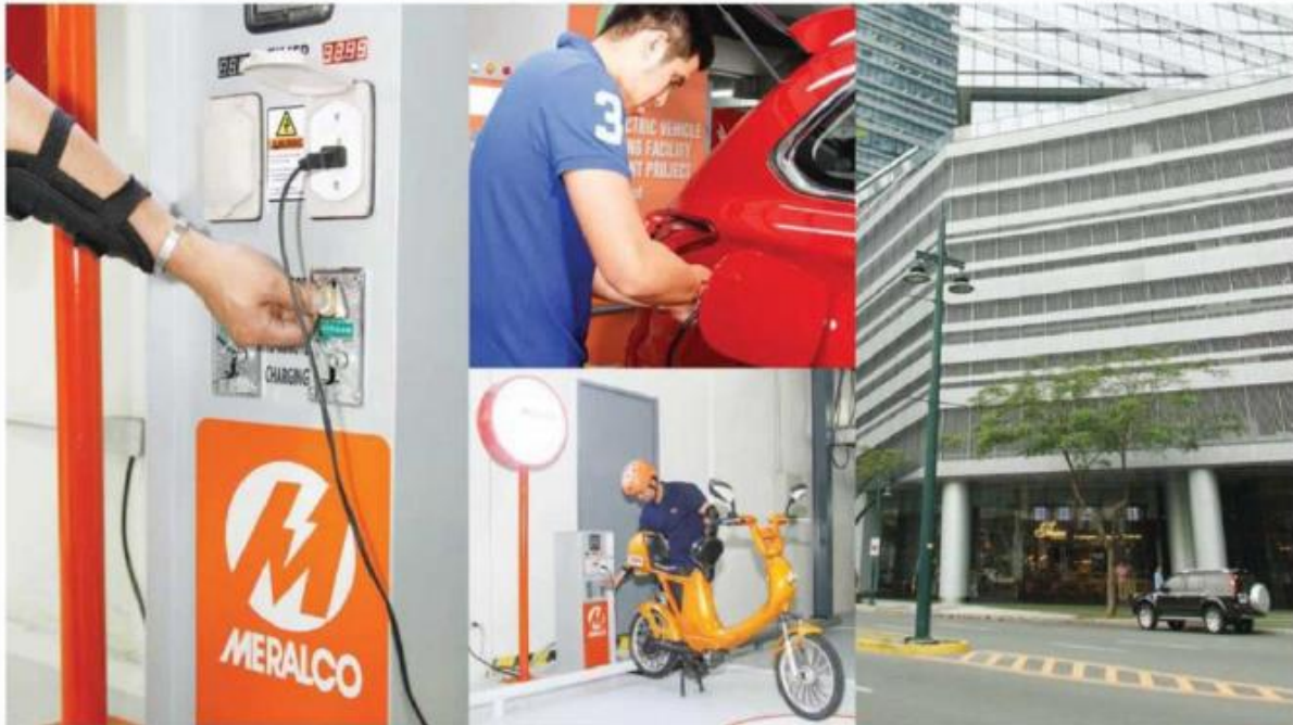
Newly-installed EV charging station at Net Park, Bonifacio Global City makes use of coin-operated charging pod.
