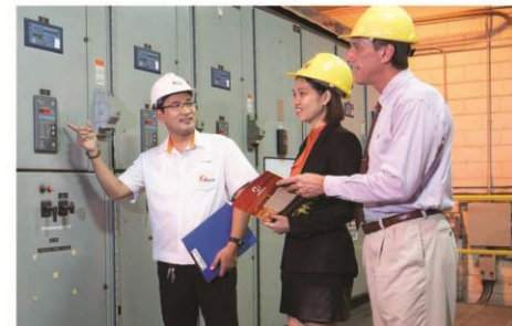
Miescor representative Antonio Lopez (left) and Meralco Relationship Manager Joy Mendoza (middle) are accompanied by US Embassy Senior Facility Manager Paul Schaefer during an on-grounds electrical facilities inspection.
